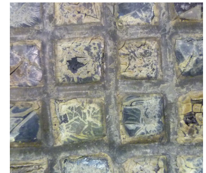
Failing viacryl application - detail Bourges Cathedral
